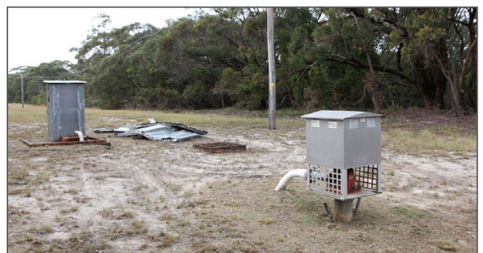
Figure 2: Tomago bore & pumping station owned by Hunter Water (source: Hunter Water)
