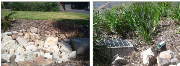
Figure 11: Left: Infiltration basin located in the front yard. Right: overflow pit with grate and inflow pipe (source: HCCREMS)
