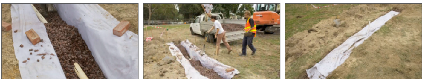
Figure 5: Construction of an infiltration trench at Stringy Bark Creek, Victoria. Source: Melbourne Water (2010)
