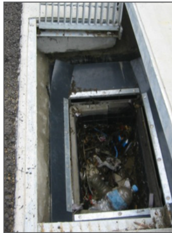
Figure 9 – accumulated sediment and rubbish requiring removal (source: Storm Consulting)
