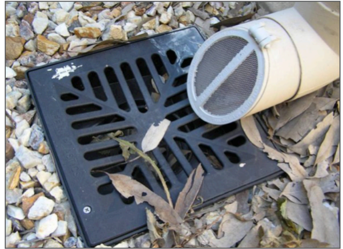
Figure 12: Clean inlet screen in tank. (Photo courtesy of Lake Macquarie City Council)
