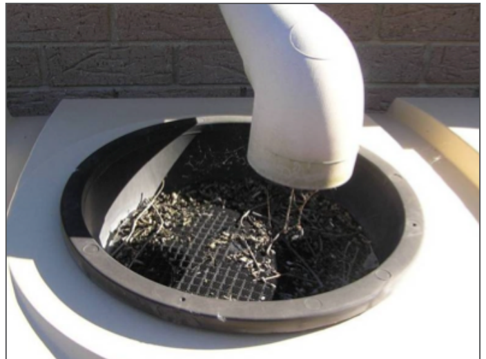
Screen over the inlet at the top of the tank
