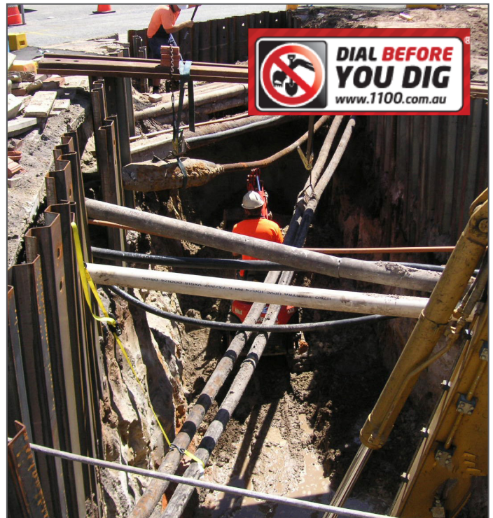
Figure 4: Excavation pipes that can significantly impact on Water Smart designs. (Source: RA SMIth Contracting).
