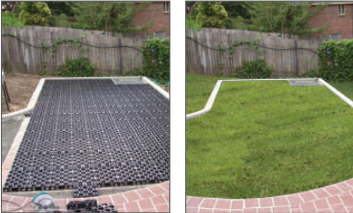
Figure 12: Runoff storage units under a courtyard and garden during installation, and after (Image source: Atlantis)
