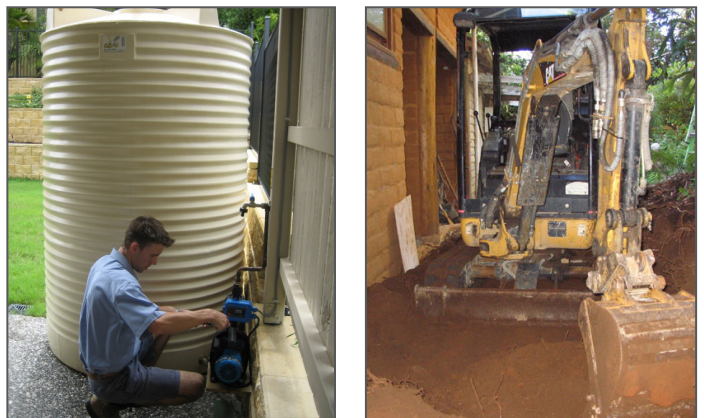
Figure 13: Maintenance activities can range from regular inspections (left) (Source: New Age Plumbing) to one-off tasks on large developments that may require specialised equipment (right). (Source: Micro machine earthworks).
